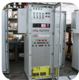
Inlet & Outlet DeNo x Alstom Power Group
