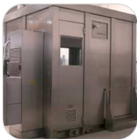
Shelter EEx p Refinery ENI Group
