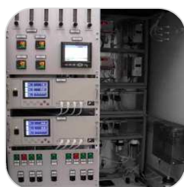
Double Streams CEMS during cabling
