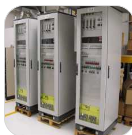
Multiple CEMS Hellenic Petroleum
