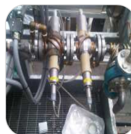
2 streams OIW FPSO Aquila ENI Group
