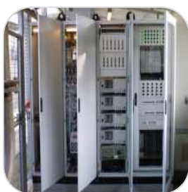
Four Streams Cogeneration Plant
