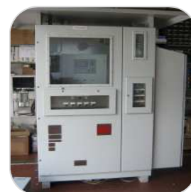
Zone 1 Eex p Calorimeter General Electric
