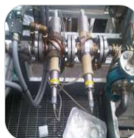
2 streams OIW FPSO Aquila ENI Group
