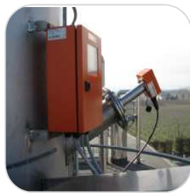
Stack Ultrasonic Flowmetering
