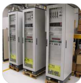
Multiple CEMS Hellenic Petroleum
