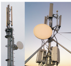
GSM/CDMA tower base stations
