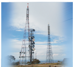
Rural Telephone Exchanges
